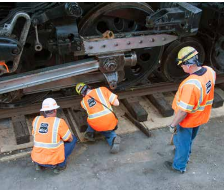
The steam crew checks the position of the No. 1 driver wheel on temporary track as it inches out of its museum berth. Plywood under the ties was installed to keep level on undulating parking lot surface.
