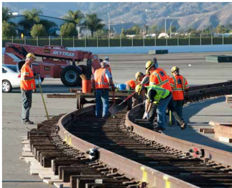
Building track in the parking lot of the Los Angeles County Fairgrounds, the UP steam crew fashions a curve for Big Boy No. 4014 to traverse as it makes its way out of the Rail Giants Museum in Pomona, Calif.
