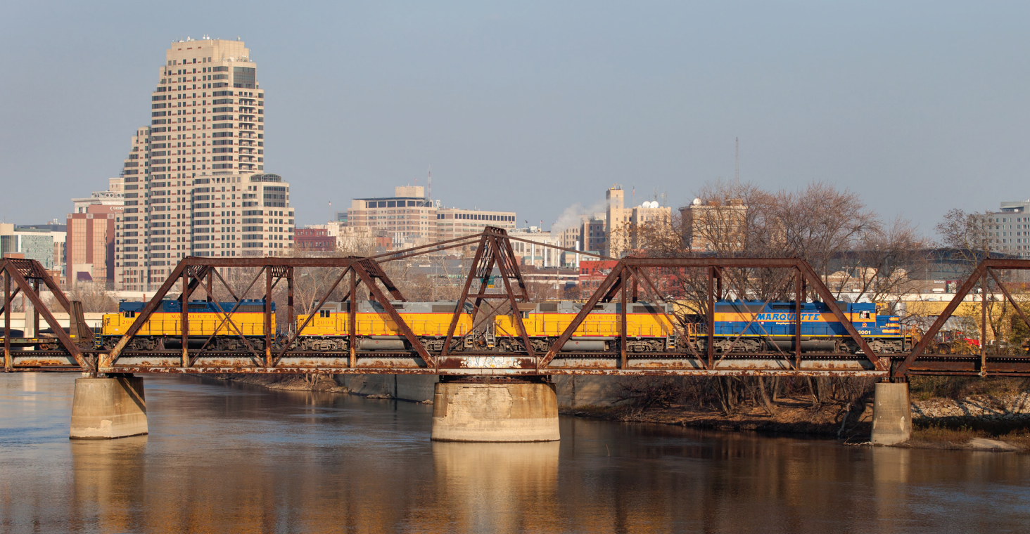
A Marquette Rail train crosses a Pratt truss swing bridge over the Grand River in Grand Rapids, Mich., in 2012. The 180-foot rim-bearing span, built in 1903 by the Pere Marquette, only served as a moving bridge for a few years following its installation. James Guest
