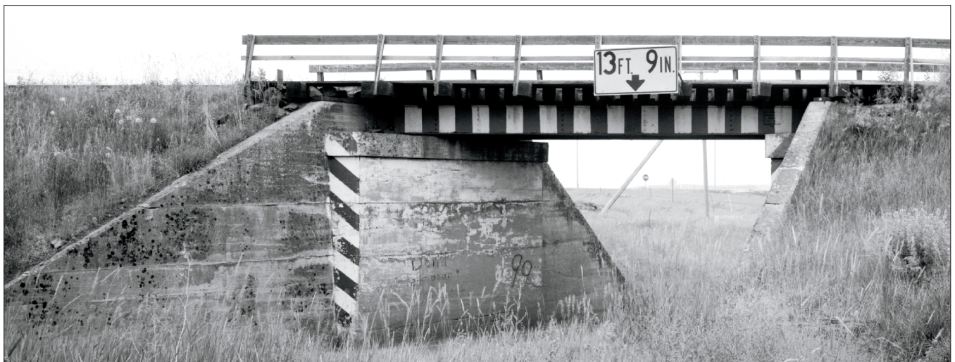
This simple skewed-end beam bridge over a gravel road on the Camas Prairie in Idaho is supported by a simple concrete breast abutment with tapered wing walls that match the fill behind them. Also note the warning stripes (on both the wall and beam) and sign. Glenn Rudolph, Historic American Engineering Record
